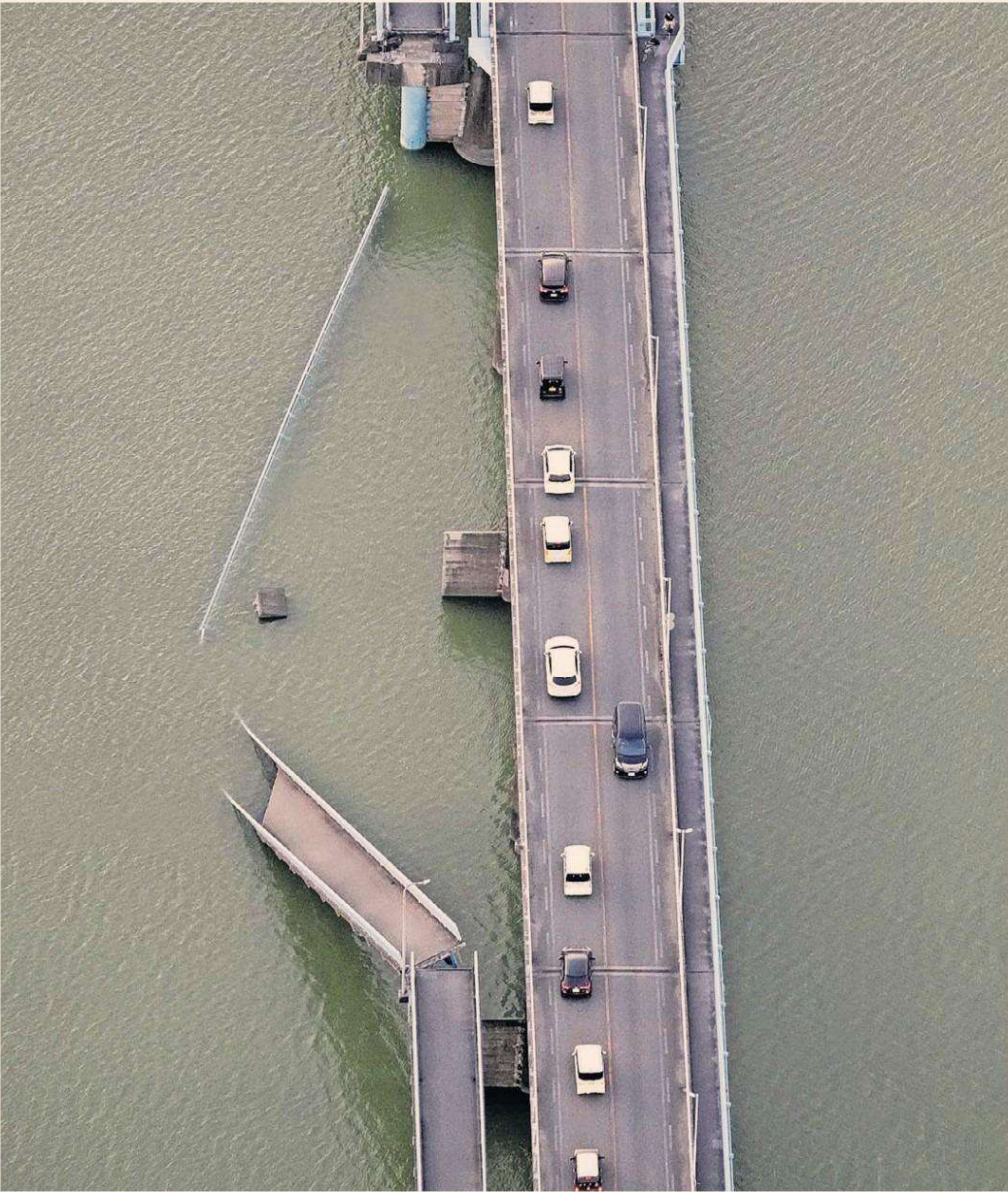
Part of a bridge that collapsed after the earthquake in Yatsushiro in Kumamoto prefecture — Kyodo News via AP
